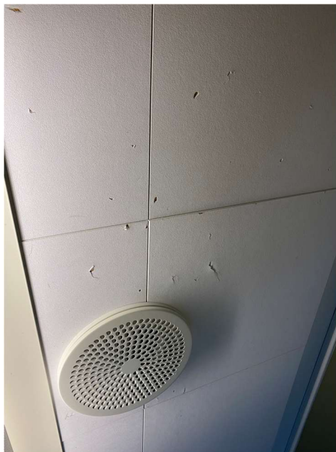
25 Dekker. Skadet himling.
