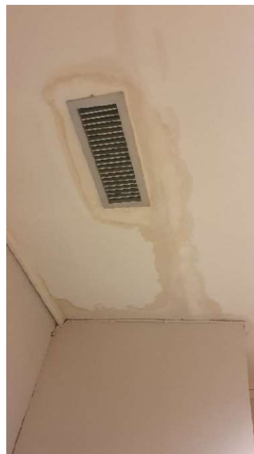
26 Yttertak, himling i korridor i plan 2
