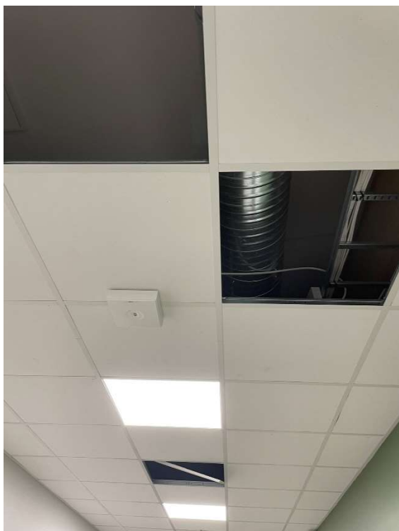
25 Dekker. Manglende himlingsplater i gang. Monter nye.
