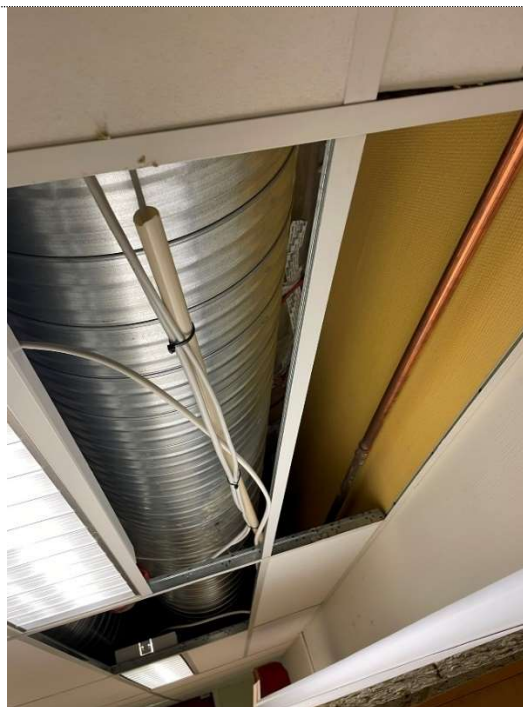
25 Dekker. Manglende himling inni klasserom.
