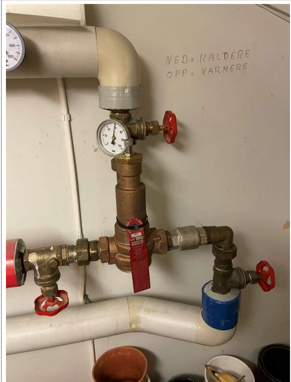
32 Varme. Mangler merking.
