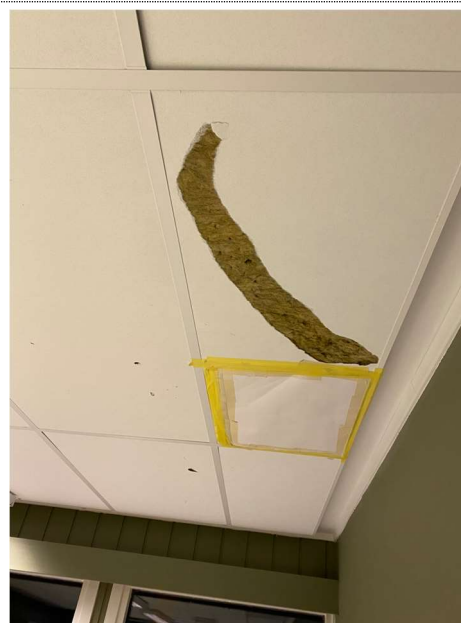
25 Dekker. Skadet himling.
